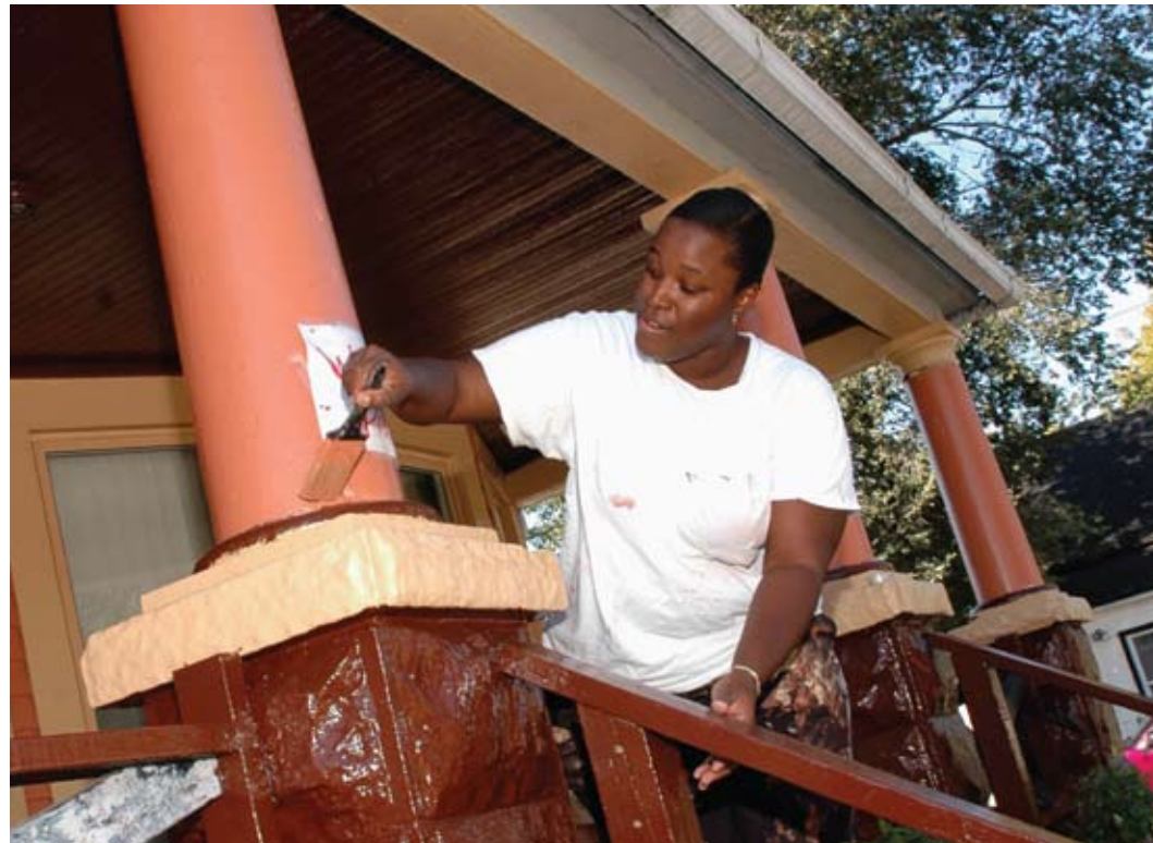
Residents improve their homes in target neighborhoods where NPI is helping to renovate vacant homes and return them to the market.
