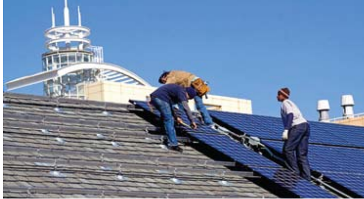
Workers from Evergreen Energy Solutions (formerly Ohio Cooperative Solar) install solar panels on Case Western Reserve University. (Photo credit: Janet Century)
